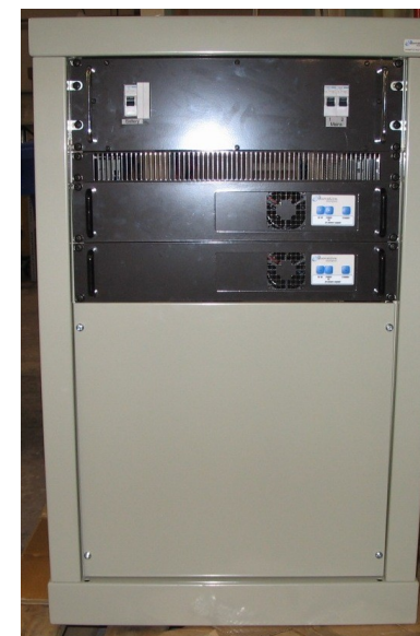
Cabinet with MCBs, No-Break DC power supplies with batteries behind bottom panel
